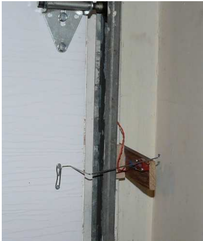
The door contact installed at the garage door.
